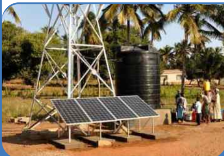
Drinking Water & Sanitation
